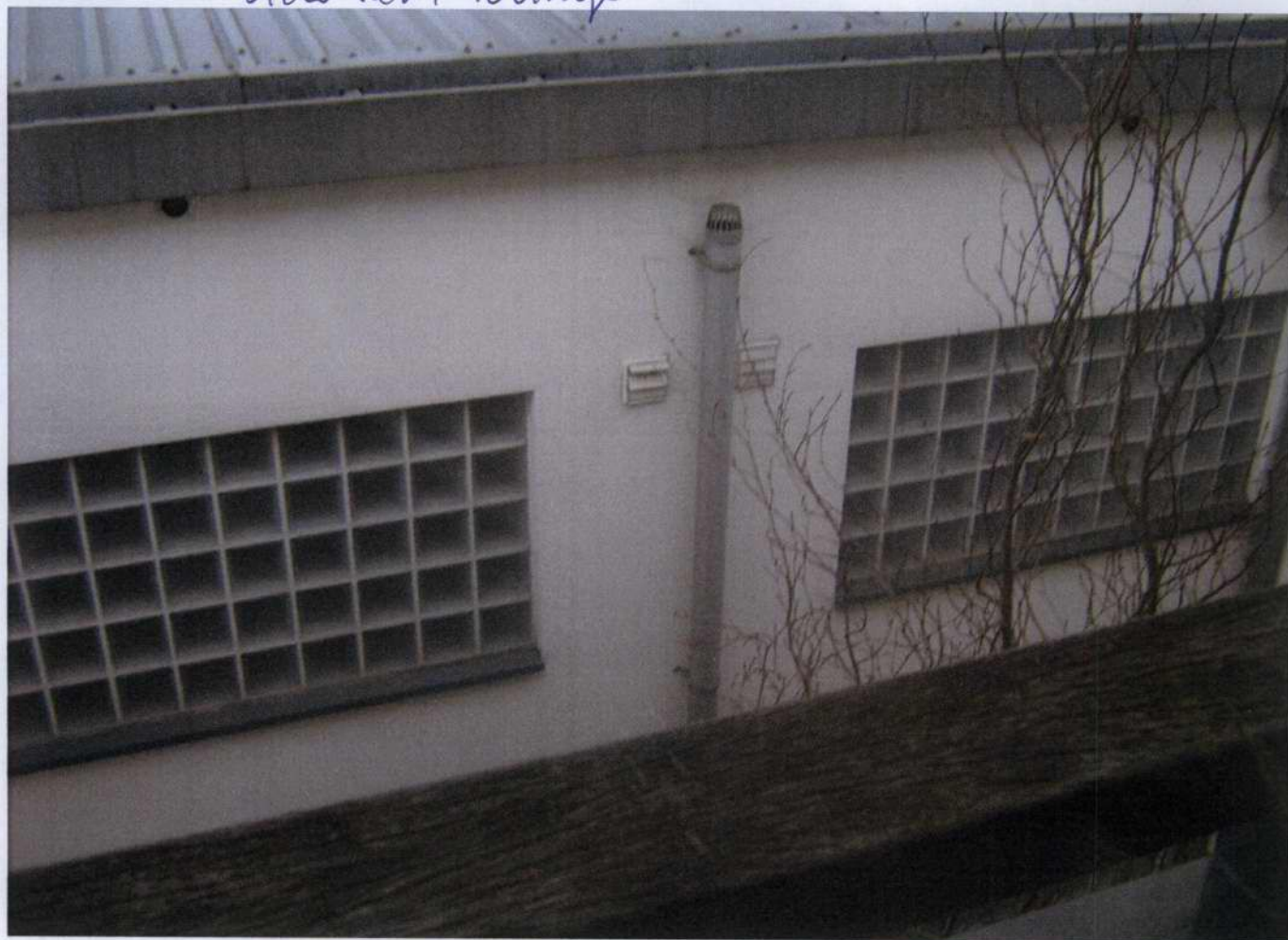
glazed brick to kitchen in flats at first two below. internal courtyard.
